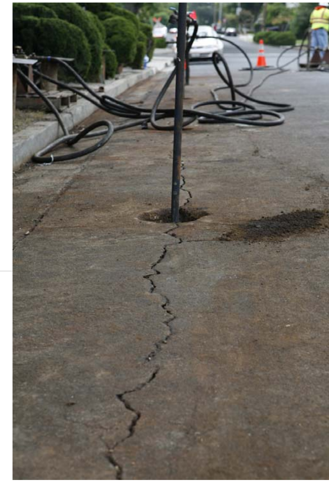
Frac casing alignments in park and street
