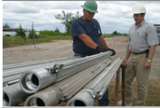
Chad Givens, GeoSierra site manager inspects specialized bore hole casings with Scott Bowen, Environmental Management Directorate hydrogeologist and project manager. (Photo by Brion Ockenfels)
