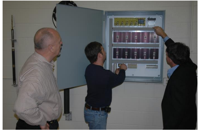
GeoSierra's Seismic Switch & Electro-Osmosis Control System Installed at Ground Floor Level of Office Building
